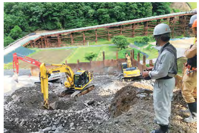
Allows for remote control at dangerous worksites
