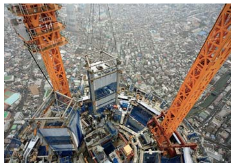
Mounting a section of steel frame attached with safety equipment by a crane
