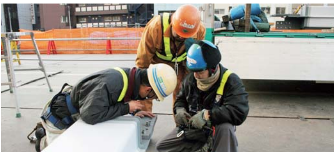
Carefully checking a steel frame to make sure it was processed and delivered as instructed
