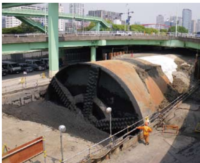
The slurry-type shield machine, measuring 13.6 meters in outer diameter and weighing 1,500 tons, as it resurfaces at the exit-end
