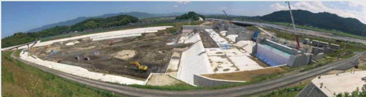
The bifurcation weir diverts part of the river to the floodway while slowing the flow from upstream (upstream is to the right)
