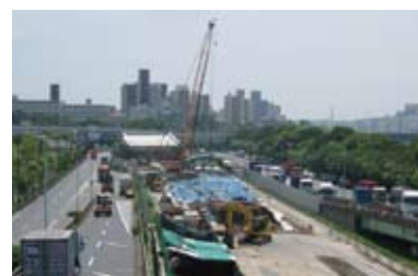
A depiction of the work in progress. The construction site was a narrow strip of land sandwiched in between two heavily traveled roads.
