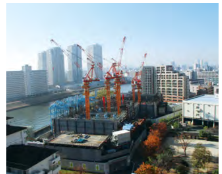
Senju Sekiya Pump Station
