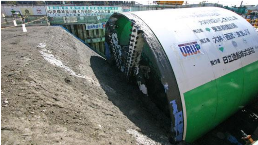
(The shield machine (TBM) launches from the ground level through the URUP method)
