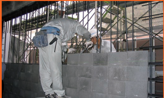
After piling up blocks while placing reinforcing bars, the wall was integrated by using special grout poured to the blocks
