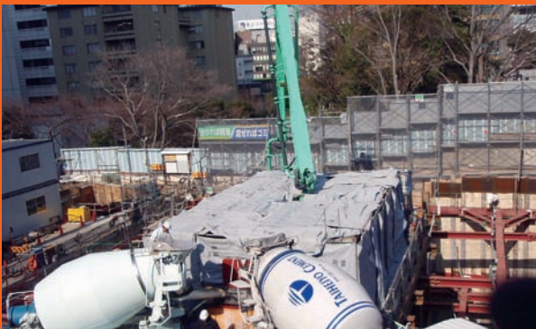
At project sites in residential areas, concrete pumps are covered with sound-proof sheets to reduce noise
