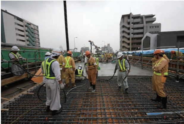
Casting concrete into the renewed floor formwork Pre-tested lightweight concrete was used
