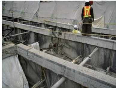
Distorted steel bridge beams by intense heat
