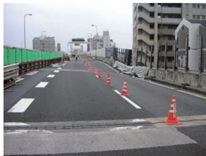
Right after the fire Deflection caused by intense heat from underneath
