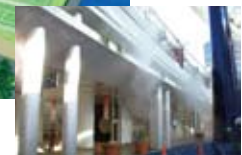
Outdoor moisture droplet cooling system
